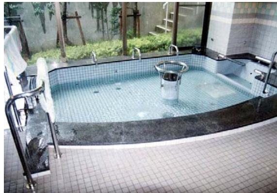
Jacuzzi after installation
