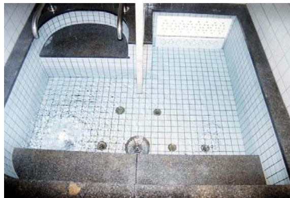
Jacuzzi after installation
