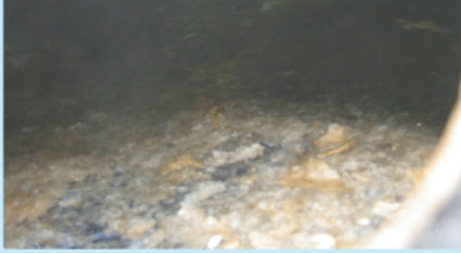
Scaling and slime build up of 16 years
