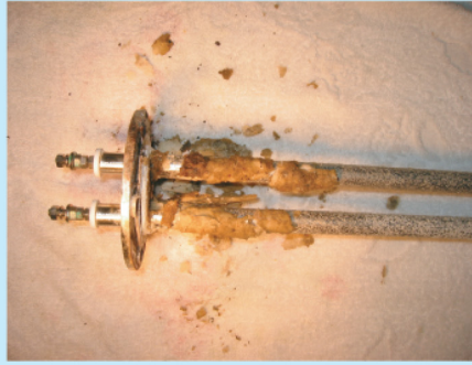
Red rust adhered to the heater section (heater is used for 16 years)
